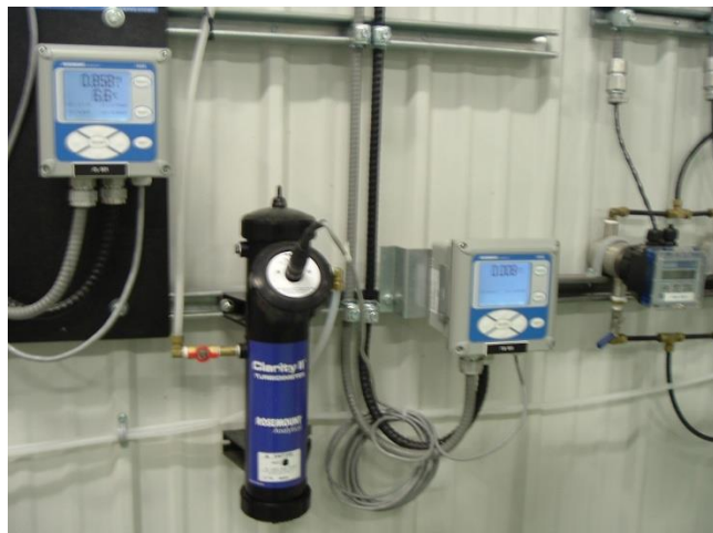
Online Monitoring Equipment
