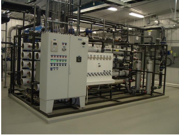
The South RO (original unit)
