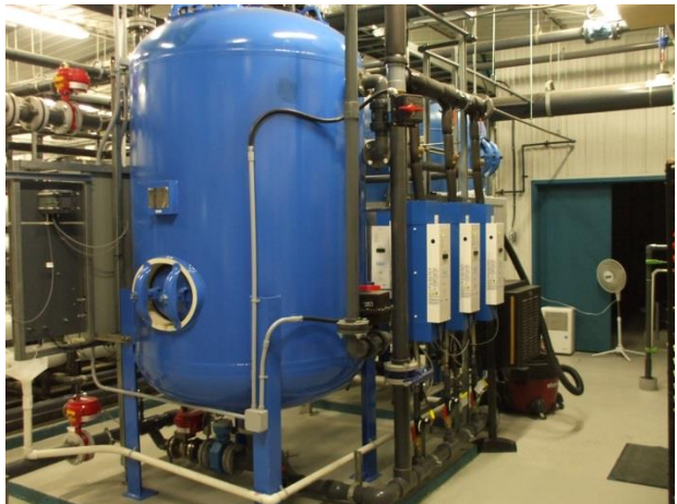
The New Sand Filter with UV
