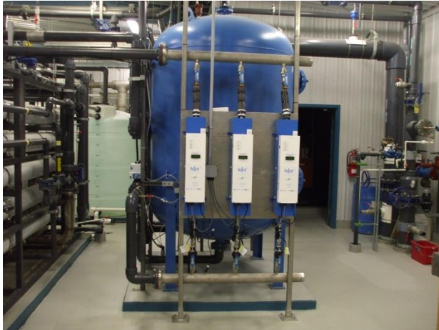
The Original Sand Filter with UV upgrade
